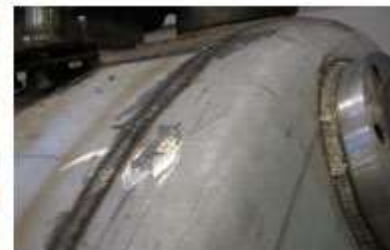
Figure 3. The knuckle of a stainless steel pressure vessel head that has been in service.
