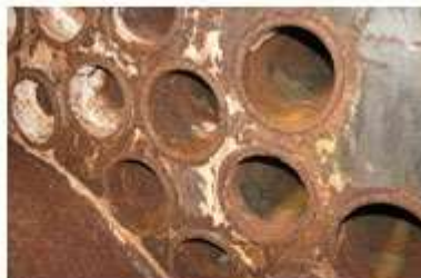
Figure 2. The tubesheet of a boiler that has been in service.
