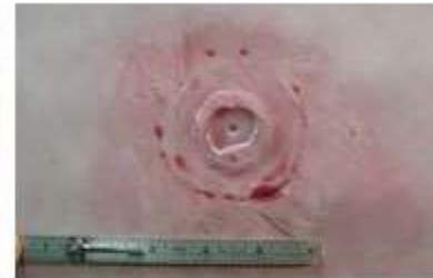
Figure 6. Evaluating indications in the spin hole plug weld. Most of the dark red indications are rejectable defects per ASME Section VIII.
